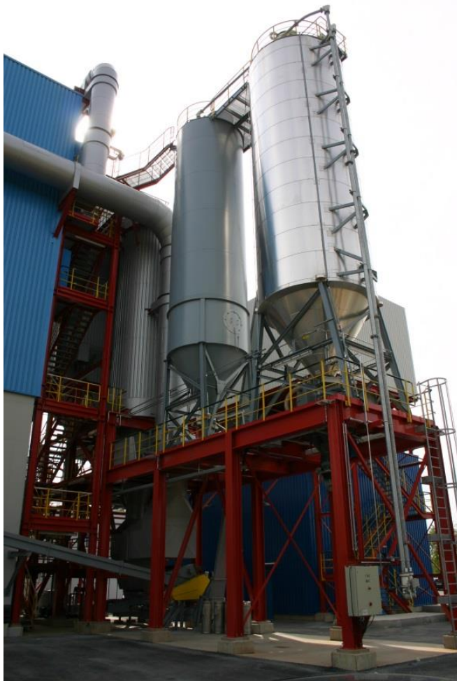
Plate 3.11: Typical Storage Silos
